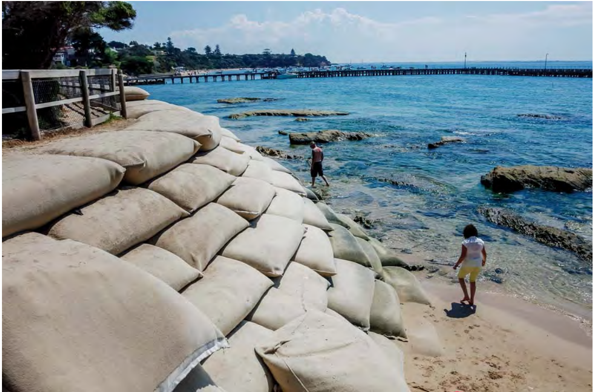
Figure C-7 Eroded beach in front of a geotextile container seawall
